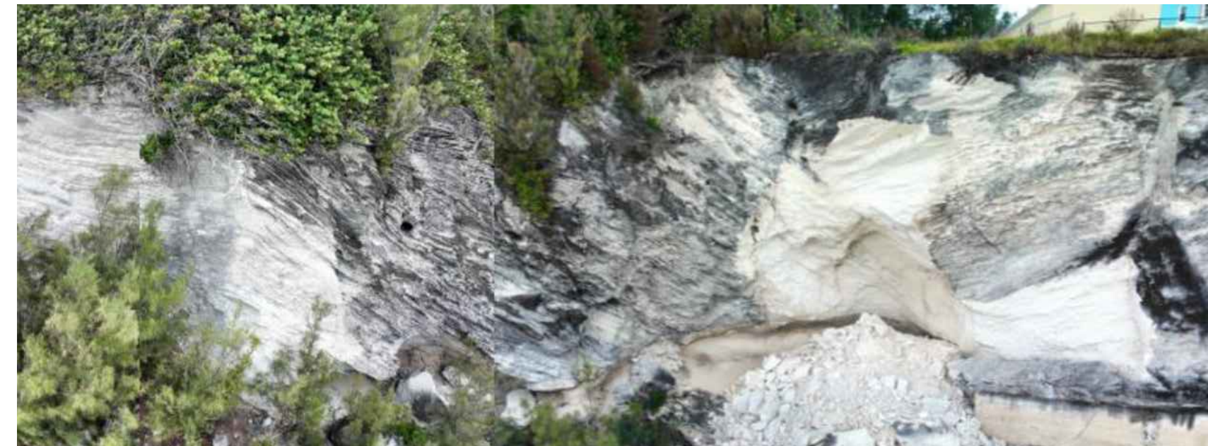
FIG-1.12 SECTION OF EXPOSED CLIFF FACE DIRECTLY BELOW THE PROPOSED EVENT LAWN LOCATION. ALL CASUARINAS TO BE REMOVED AND THE ROOTS PAINTED WITH TORDON OR EQUIVALENT. 2 PROCKETS OF CLIFF COLLAPSE WILL NEED REVIEW PRIOR TO ESTABLISHING THE SETBACK FROM THE EDGE.
